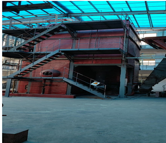
10t/h 燃煤锅炉 2
