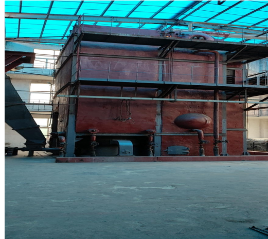
10t/h 燃煤锅炉 1
